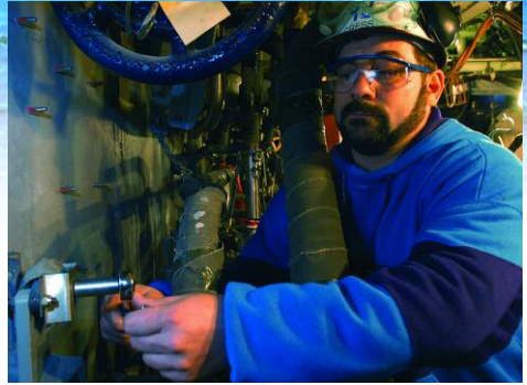
Pipefitter Wade L. Cress Jr., who was born in Concord, N.C., tightens hanger bolts.
