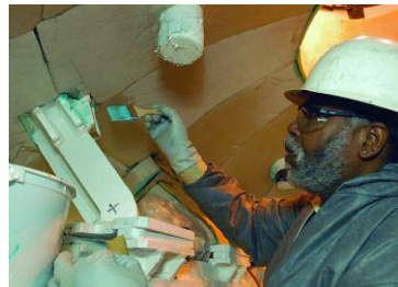
Insulator William N. Hines, a native of Edenton, N.C., applies glue to a foundation before attaching insulation in the sonar sphere.
