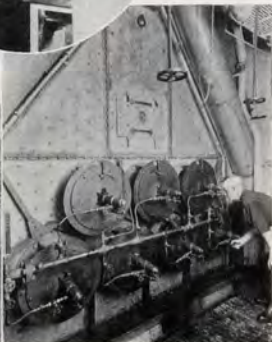
Fire room— showing front of boiler
