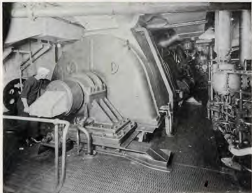
One of the two 16,000 horsepower turbo-generators
