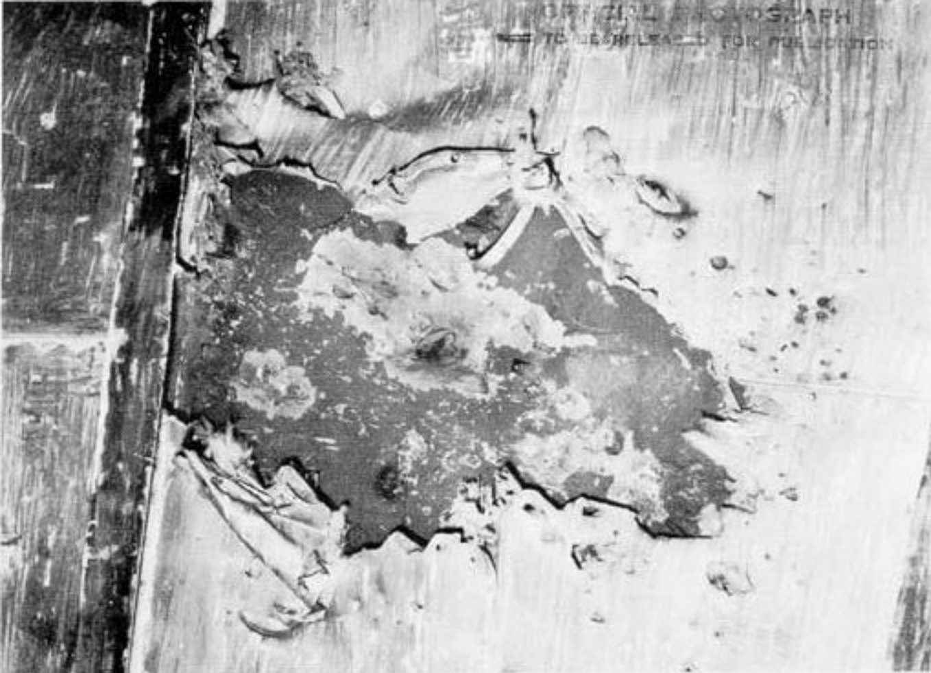
Photo 30: Hit No. 22. Damage to port structural bulkhead in battle dressing room.
