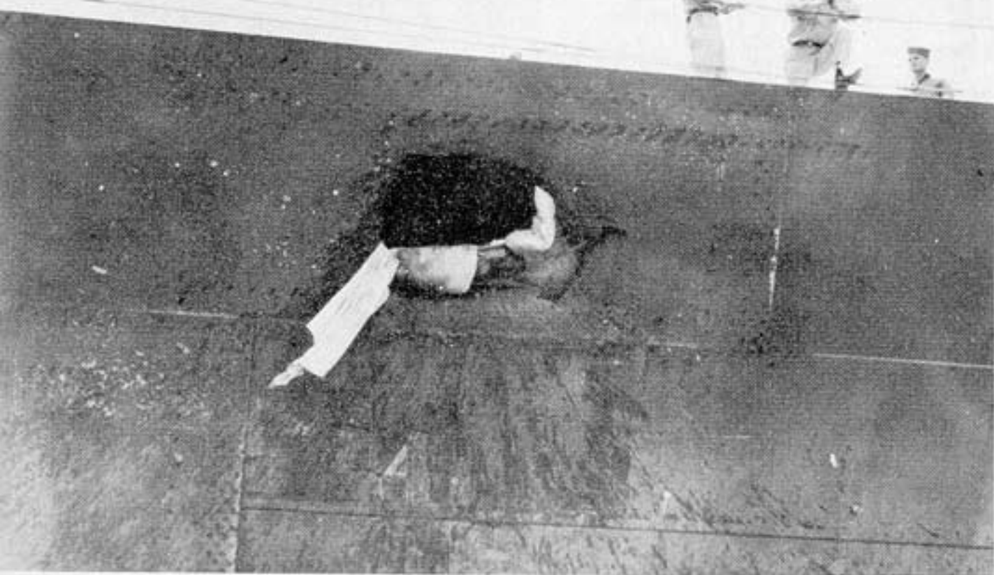
Photo 1: Hit No. 2. Hole blown in starboard sheer strake at frame 30. Note patch plates which were installed over smaller holes below sheer strake.
