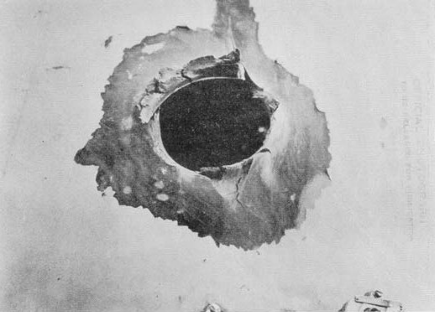
Photo 19: Hit No. 12. Exit hole in port longitudinal structural bulkhead.
